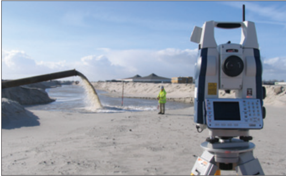
FIGURE 4: The SRX robotic Total Station at work as a six-metre embankment takes shape near Dronen. In the background, fine sand dredged from the Zuiderzee is piped directly into a prepared profile. When settled, it will provide a firm track bed for Hanzelijn's double-deck trains. (Photo: Peter FitzGibbon)
